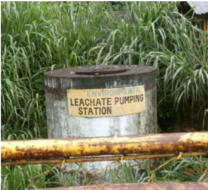
Small leachate pumping station.
