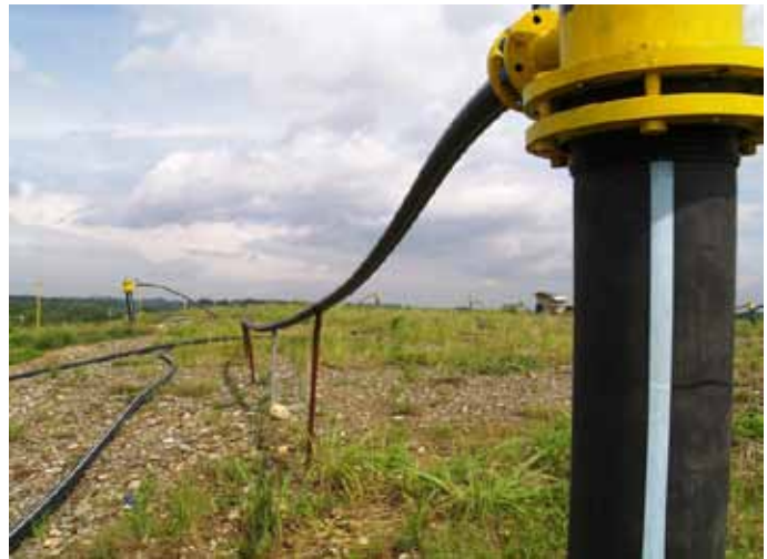
Landfill gas field.
