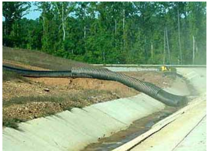
Concrete perimeter stormwater drain.
