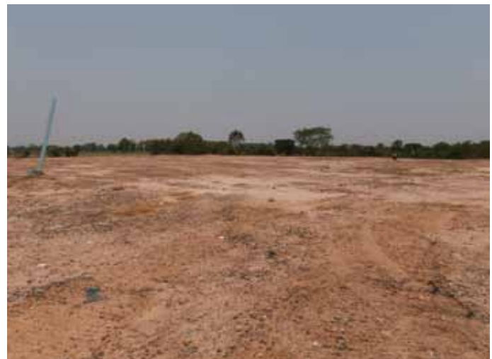
Completed section of landfill too shallow and flat.
